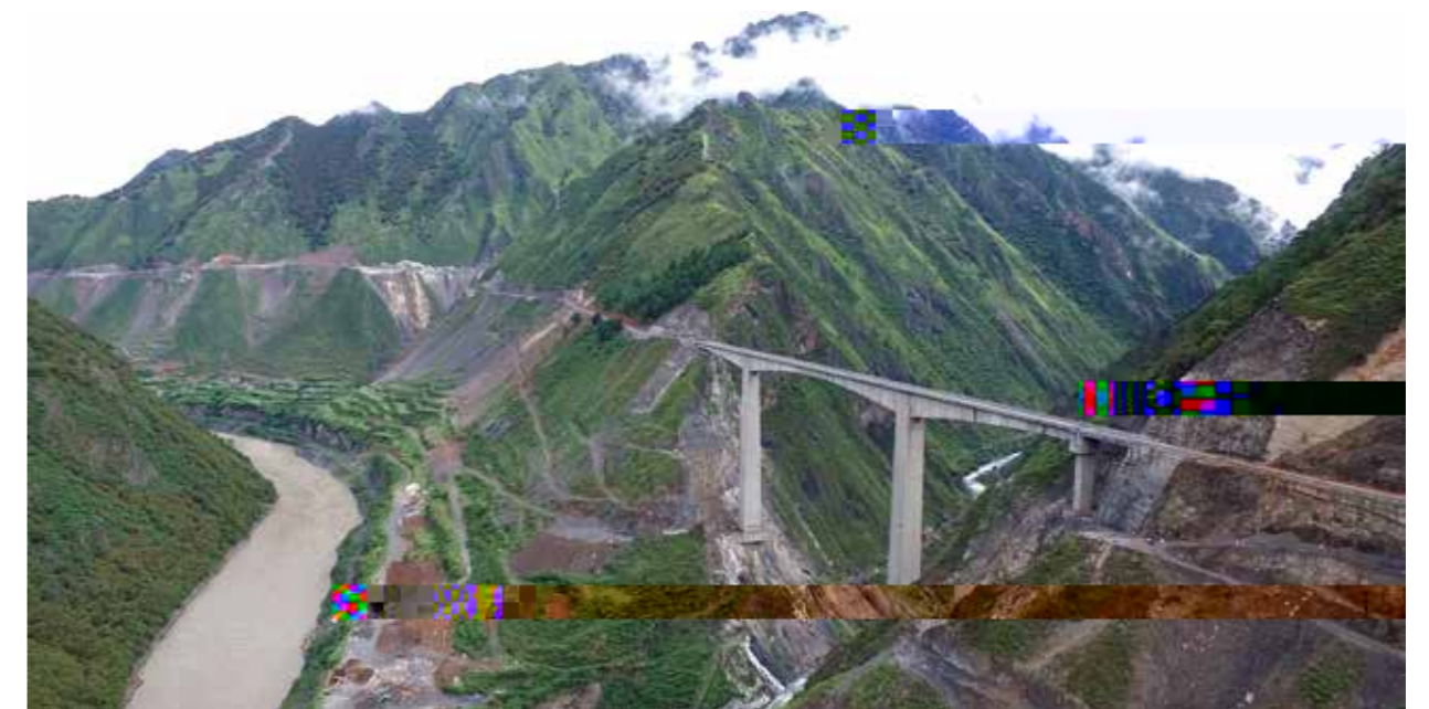
Yajiang-Xinlong Highway constructed by Yalong River Hydroin Ganzi Tibetan Autonomous Prefecture, Sichuan Province
