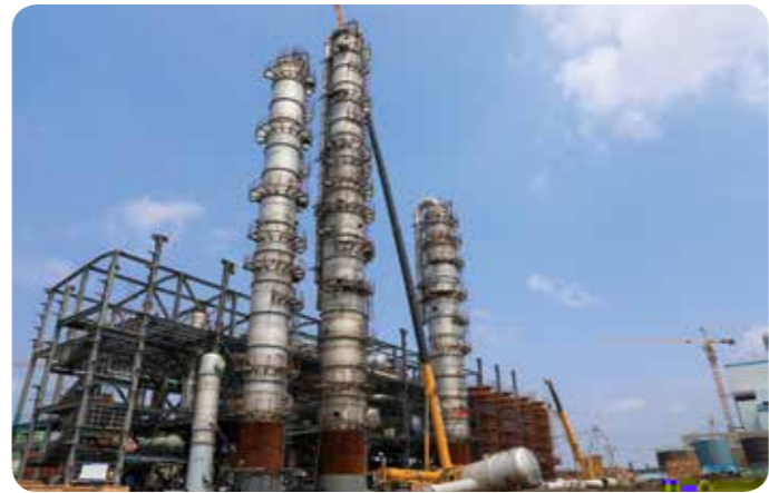
Main facility of SDIC Bioenergy Hailun Co.'s fuel ethanol project with an annual output of 300,000 tons, which now is under construction
